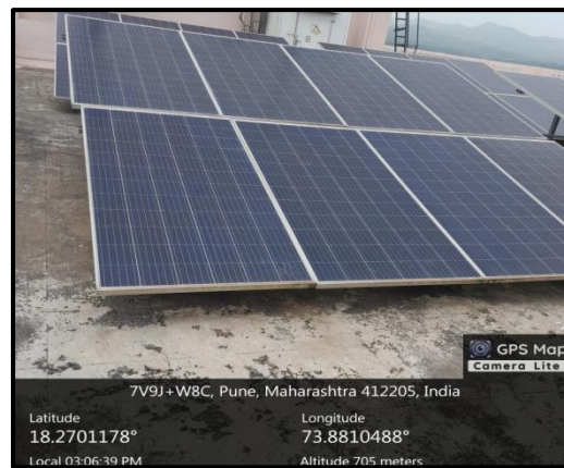
Photograph of Roof Top Solar PV Plant:
